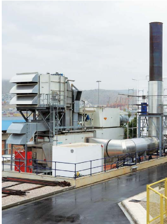
Figure II.3-3 Example Gas Turbine Package, Courtesy of Siemens
