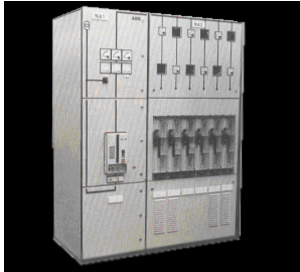
Figure II.3-7 Example of 0.4 kV Switchgear with Incoming and Outgoing Feeder Lines, Courtesy of ABB
