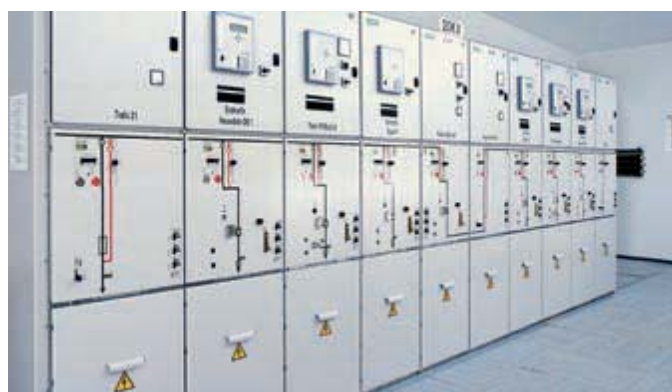
Figure II.3-5 Example of Gas Insulated Building Switch Gear, Courtesy of Siemens
