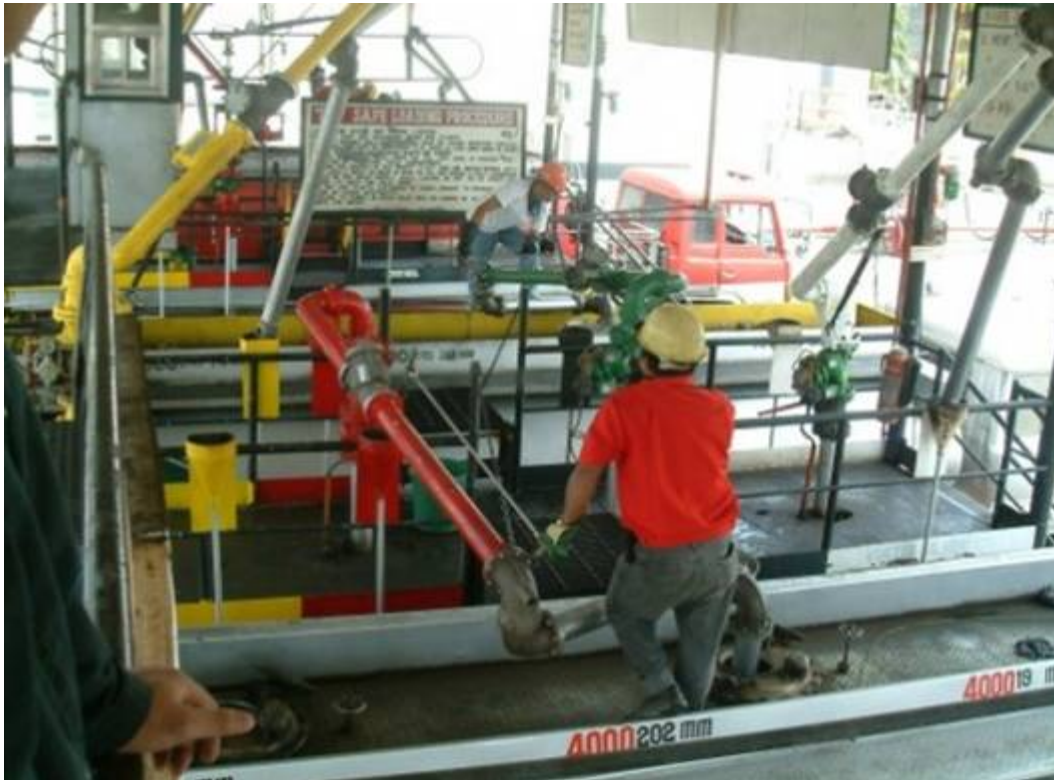
Figure II.6-7 Example of top CTMV loading facility
