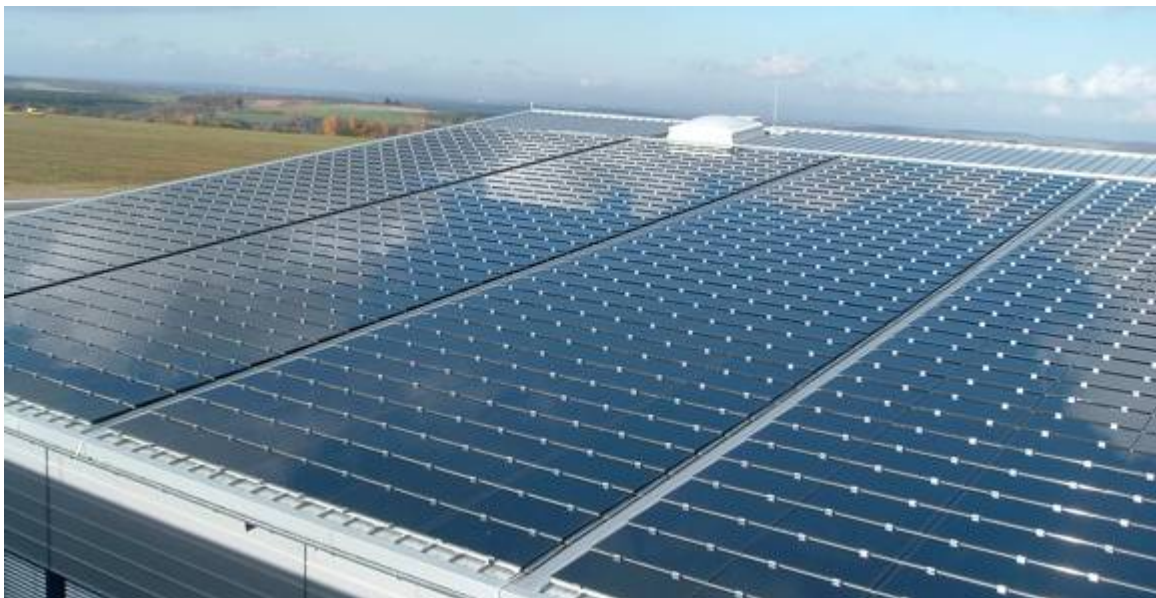
Figure II.3-9 Example of Solar Modules on Industrial Facility, Courtesy of Würth Solar
