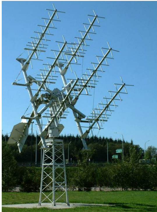
Figure II.4-2 Typical Radio Relay Antenna
